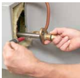
Fig. 6.5 Remove the filter and clean the limestone from all of the openings.
